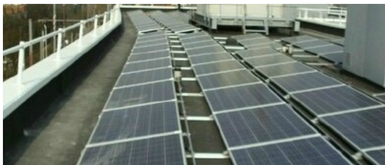
View of some of the panels installed in 2013 by GNCE as part of a 40kWp system which it is proposed to purchase
